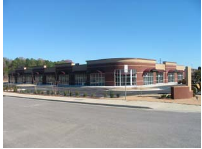
Construction continues Friday on the new Carmichael Place shopping center in Montgomery. The center is expected to open in January
