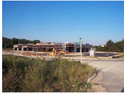
Construction has begun on a new shopping center called Carmichael Place on Carmichael Road at Woods Crossing. The site is near East Boulevard.
